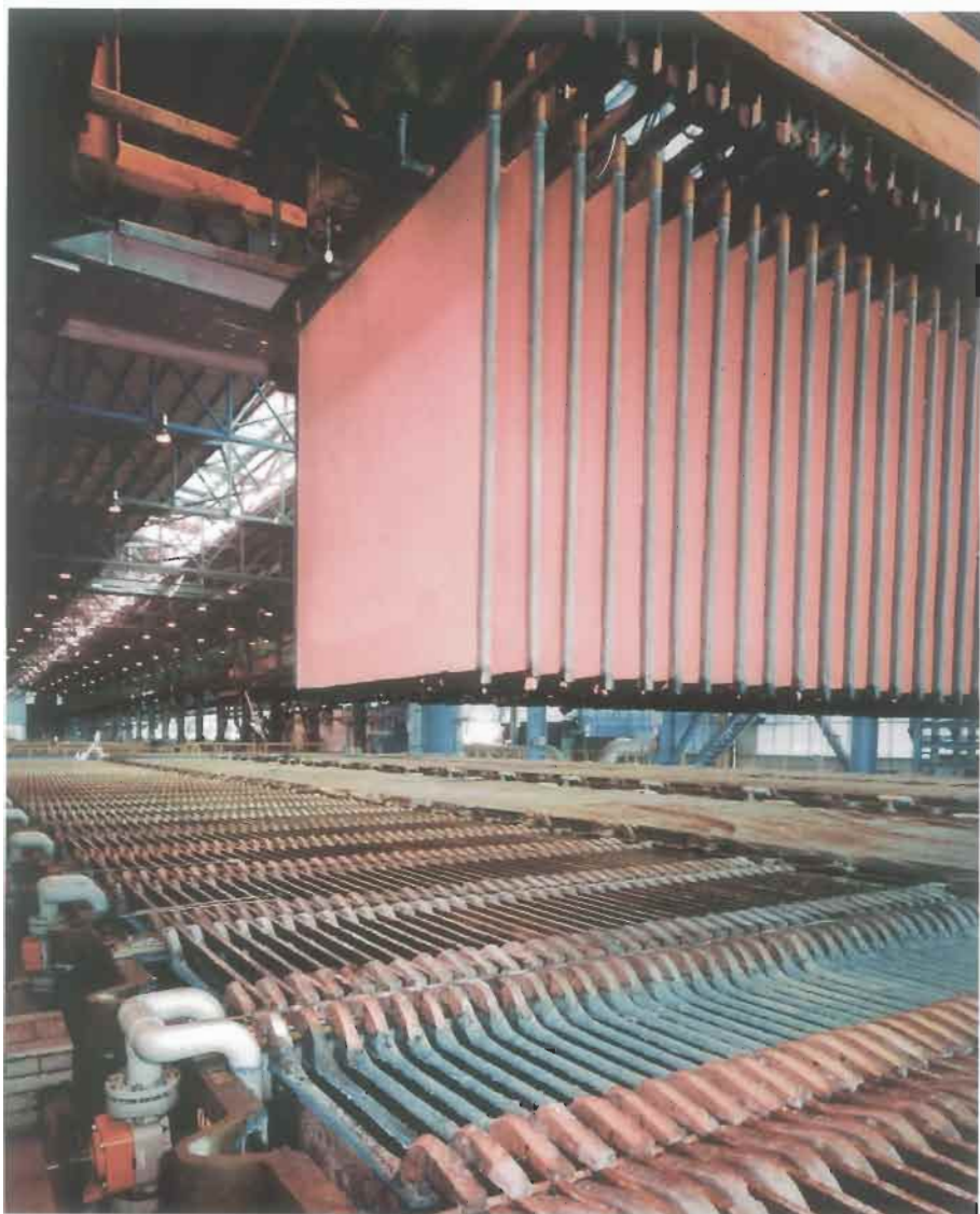
Fig. 16.0 Copper-plated stainless steel blanks being lifted from a polymer concrete cell. The cathode copper will be stripped from the stainless steel blanks and sent to market. The anodes in the cell are now 'scrap'. They will be washed, melted and cast as new anodes. The cells in the background are covered with canvas to minimize heat loss. Photograph courtesy Miguel Palacios, Atlantic Copper, Huelva, Spain.
