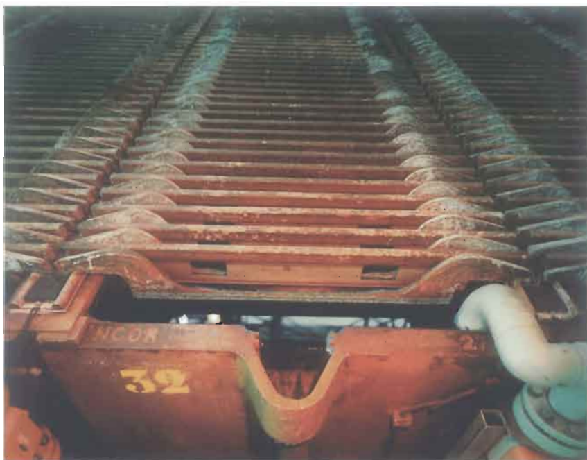
Fig. 16.2b. Copper anodes and stainless steel cathodes in polymer concrete electrorefining cells. (Photograph courtesy Miguel Palacios, Atlantic Copper, Huelva, Spain)
