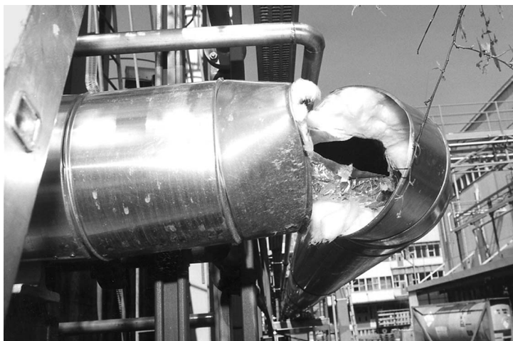
Fig. 14–1. Destroyed pipe bend
