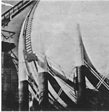
Figure 4.12 Spherical LPG Tank Insulated by Frothing-in-Place [4.54].
