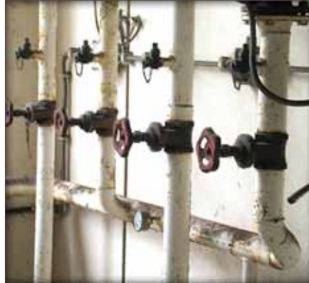
These valves don't provide critical valve and pipe information due to missing tags.
