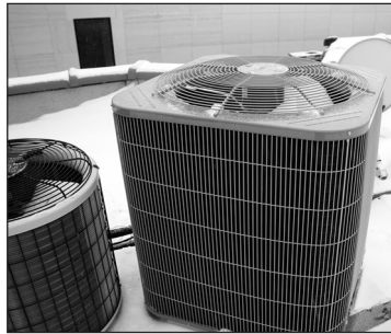
Air conditioning systems
