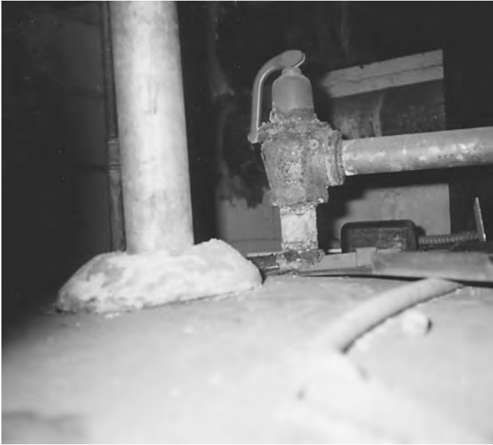
Figure 17.8 A corroded safety valve.
