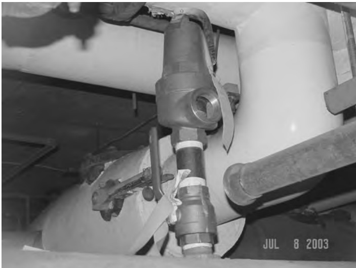
Figure 17.3 A discharge pipe is disconnected.
