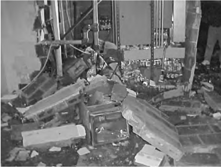
Figure 1.2 Water heater explosion at Avon High School.
