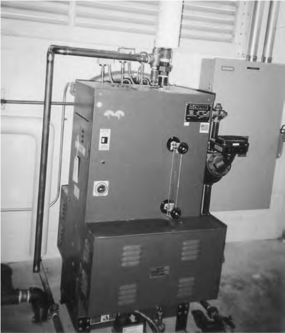
Figure 9.2 Safety valve on an electric boiler.
