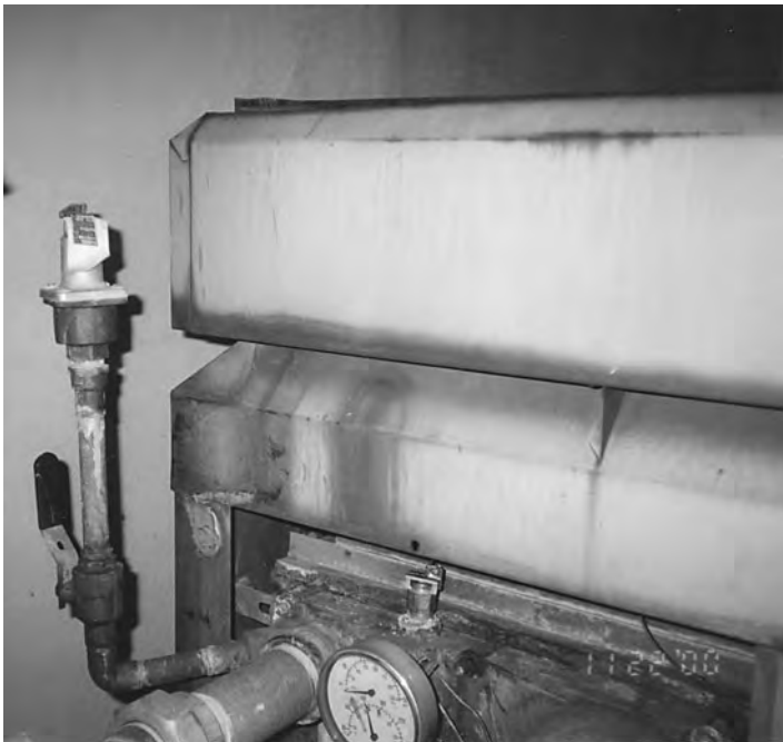
Figure 18.5 A stop valve is wrongly installed between the vessel and safety relief valve.
