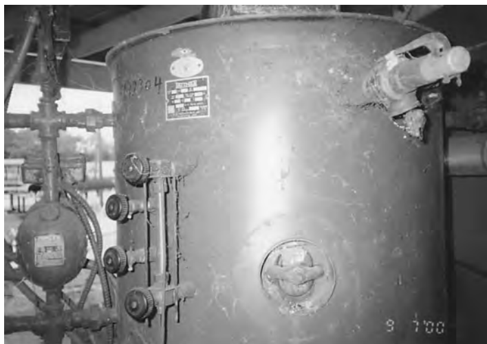
Figure 16.1 A pressure relief valve without a discharge pipe.
