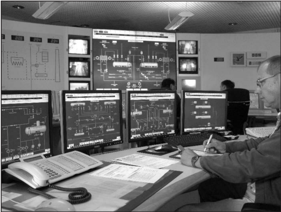
Figure 8–2 Standard layout for a modern combined cycle power plant control room
